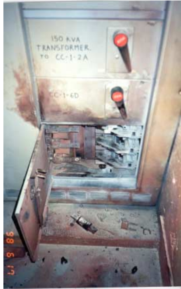
Figure 48—Low-voltage class circuit isolation equipment (top view) where Peter Wiebe was engulfed in the discharge of the arc-flash products (heat, spatter, plasma)
