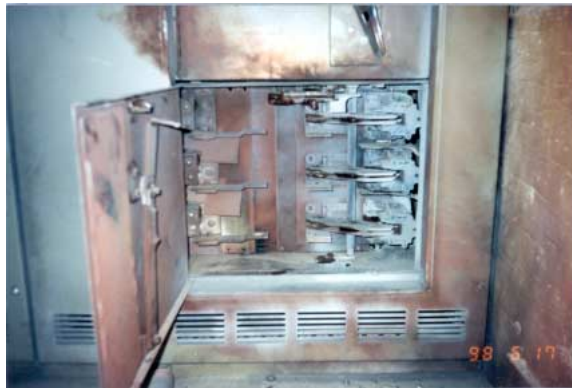
Figure 47—Low-voltage class circuit isolation equipment (front view) where Peter Wiebe was engulfed in the discharge of the arc-flash products (heat, spatter, plasma)
